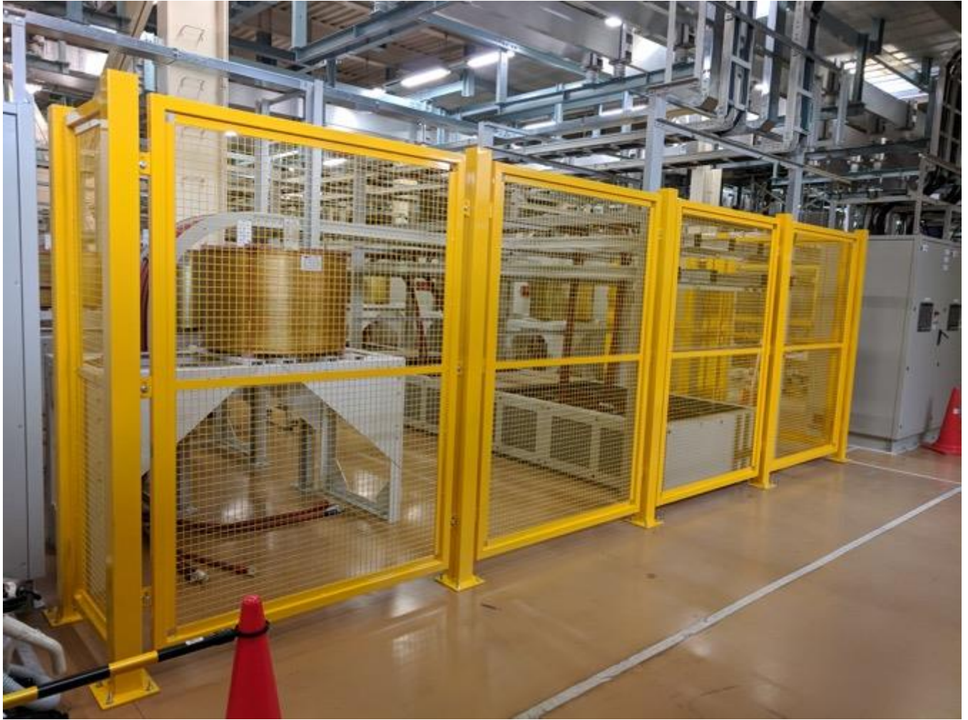
Figure 1: The installation of the power supplies procured by ENEA is essentially completed.
