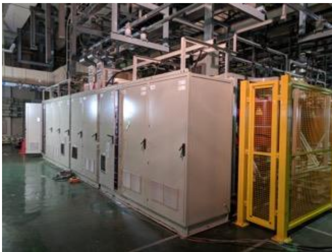
Figure 2: FPPC1 under testing
