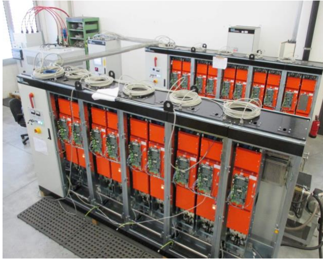
Figure 1: System at the E.E.I. premises for the routine and integrated tests of the RWM PS
