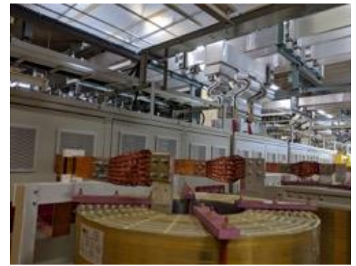
PS DC reactors and busbar connection
