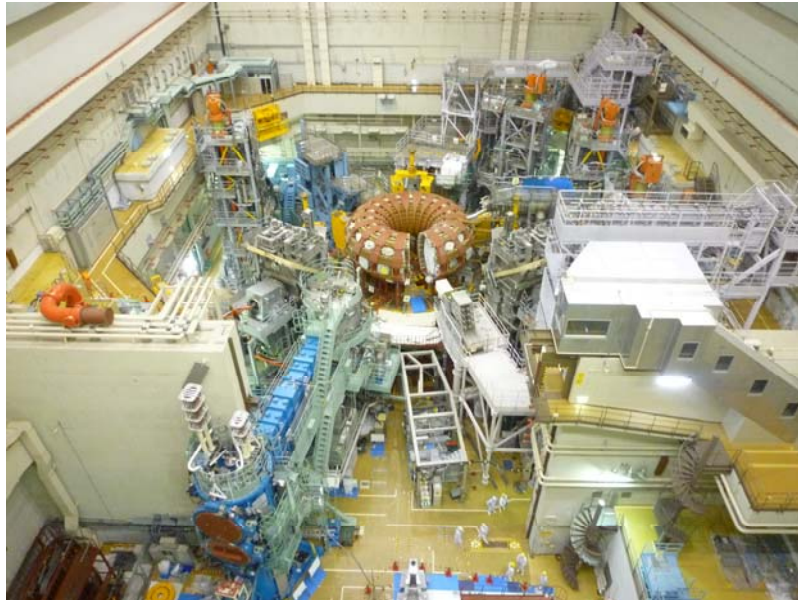
Current state of disassembly
