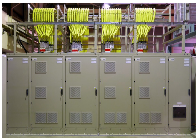
TF coil PS (front view)
