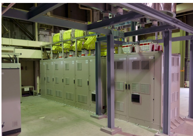
TF coil PS installed in the TF PS room
