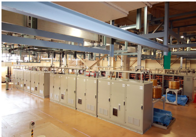
EF2 – 5 coil PSs installed in the rectifier room
