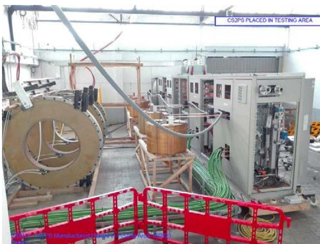
Figure 2: CS2 PS in the testing room of the JEMA laboratory
