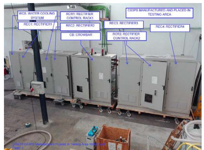
Figure 3: CS3 PS in the testing room of the JEMA laboratory
