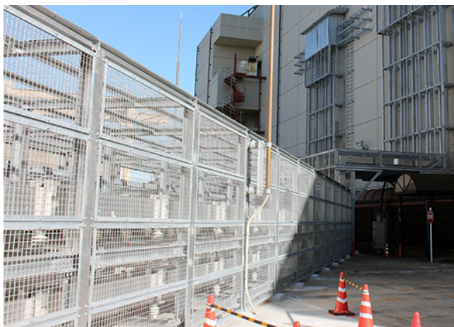
Figure 1: Safety fences mounted around the feeders
