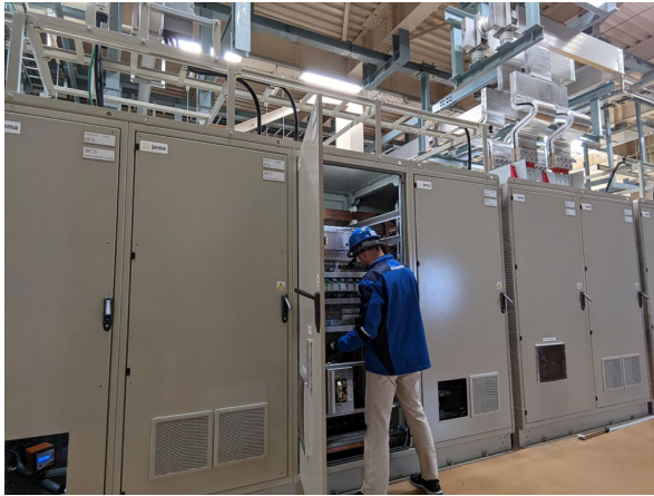
Getting remote support from Europe while checking the inside of EF3 PS cubicles
